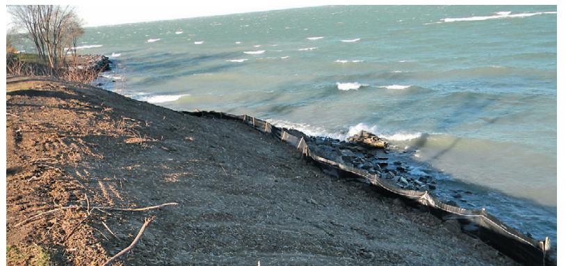
A look at the earlier shore erosion and corrective measures being undertaken by the Town of Porter on the Lake Ontario shoreline.
